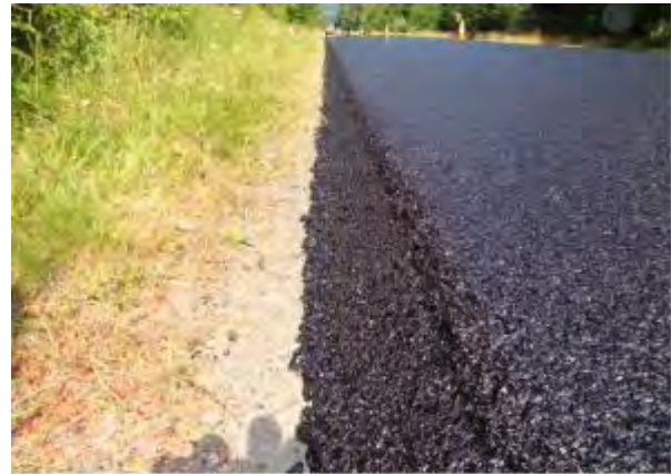
Figure 30. Pavement edge formed by the TransTech hardware prior to adding the roller. Note open texture of the HMA.
