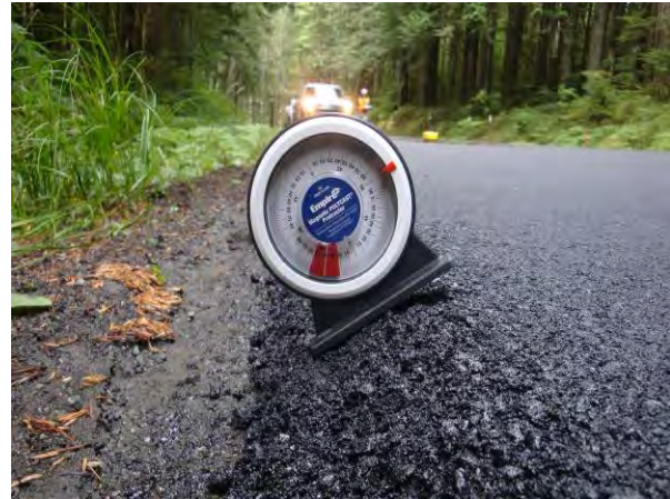
Figure 56. Slope indicator device on the edge treatment. Slope does not appear to be compacted.
