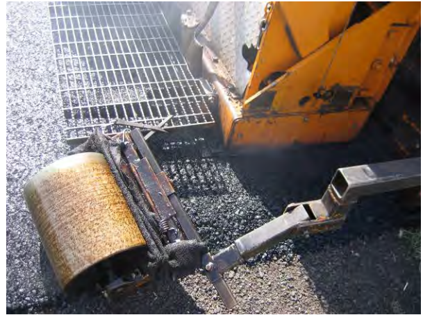
Figure 19. Close-up of roller hardware.
