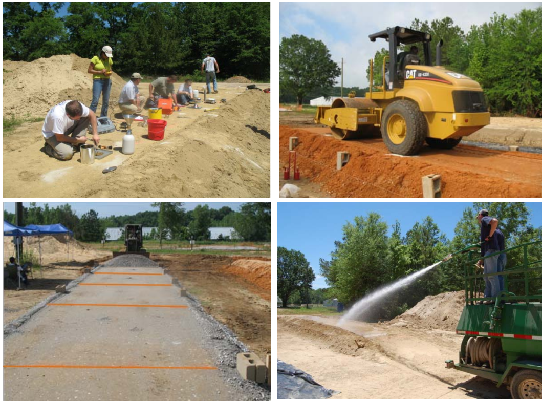
FIGURE 2 Test Execution. Top left: Device testing on ML-1. Top right: Construction of SP-SC layer (final lift). Bottom left: Construction of GP-GM with test regions marked. Bottom right: Soaking of ML-1 test section following testing of 8 th coverage.
