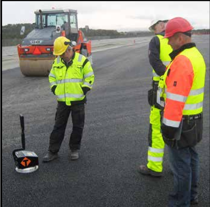
Veidekke AS paving the runway on Kristiansund airport. This is a night job in the middle of the summer, but since they are in Norway it is not getting dark there.
